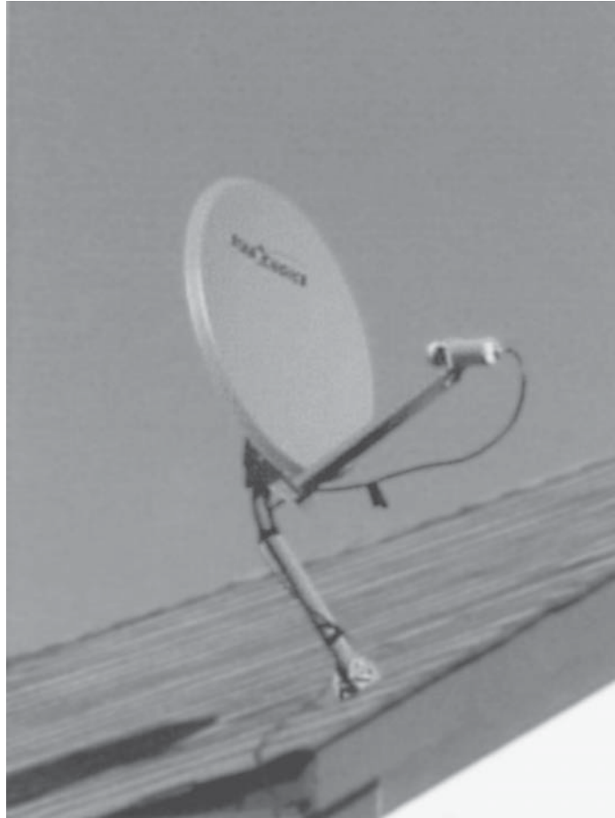
Figure 16.6 A typical DBS antenna installation.
